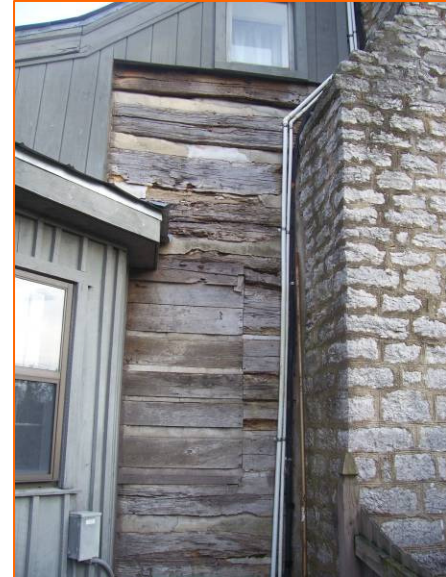
West wall deterioration. Photo by BLH Joe Cathey 1-27-2010
